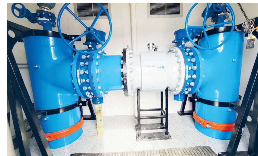
Eric Crump/H-F Chronicle The meter for the new water line from Hammond, Indiana, via Chicago Heights is several feet across.
